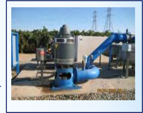
Replacement Electric Ag Pump
